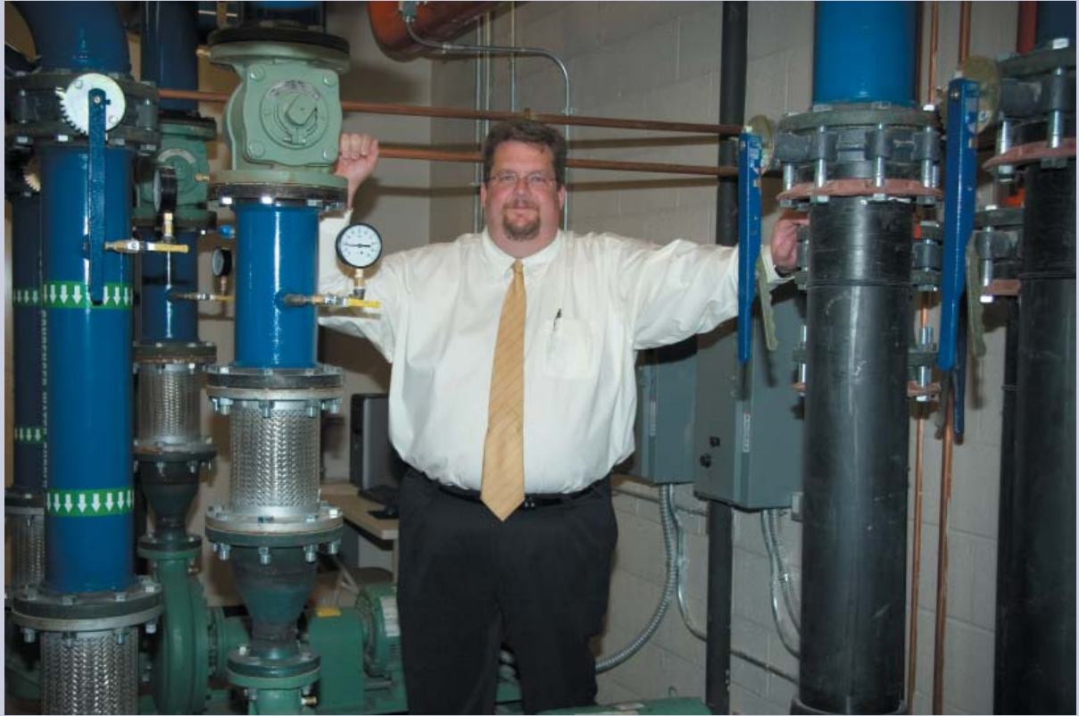
Don Johnson, director of facilities at Lipscomb, displays the equipment room.
