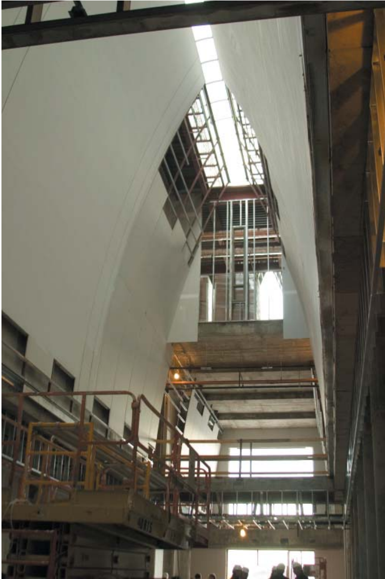
The Ezell center has large vaulted ceilings which add to the beauty of its design.
