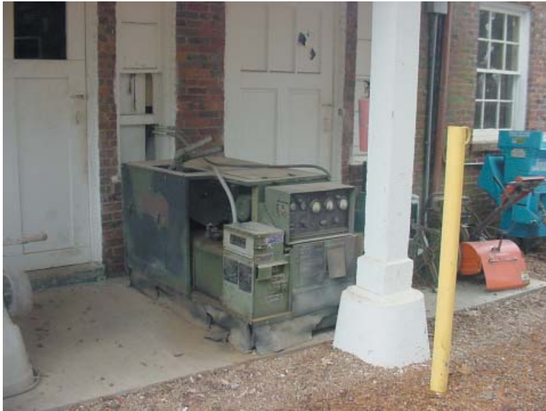
Courtesy of Nashville Electric Service.
