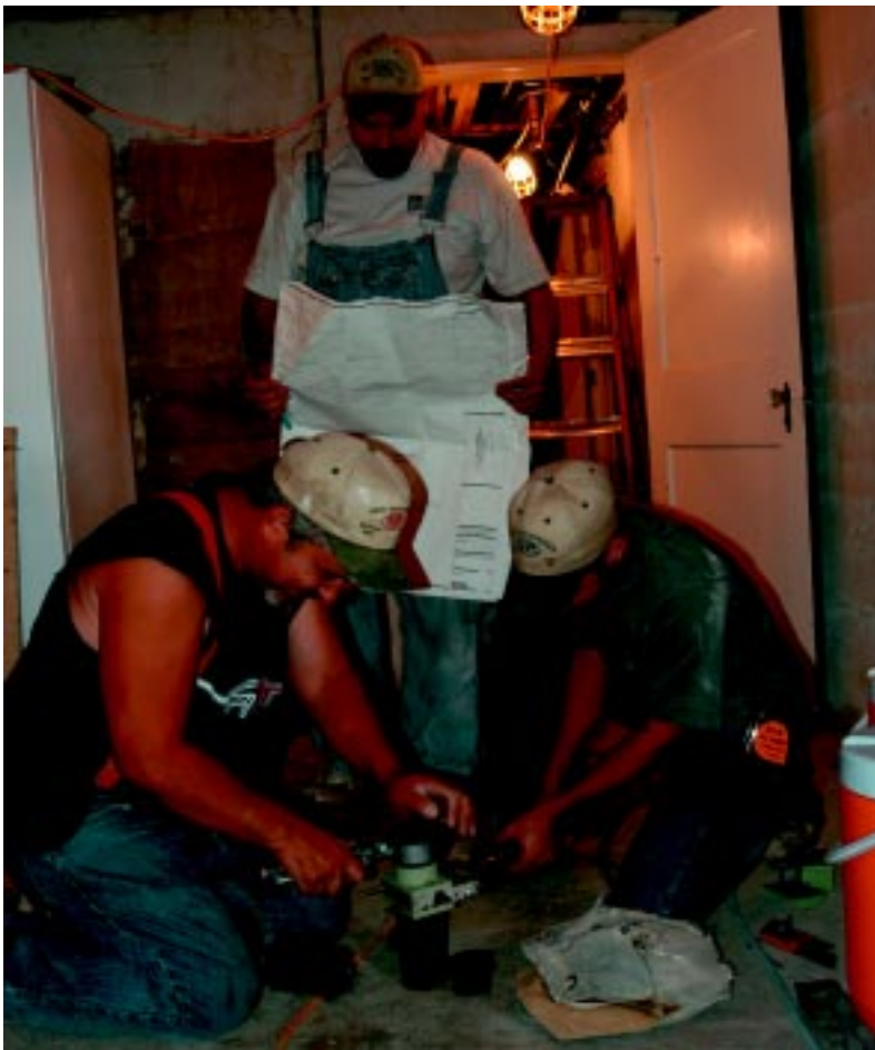
Mark Swift of Geo-Enterprises, Rick Dense of Dense Mechanical and David Carpenter of Geo-Enterprises finish a fusion project.
